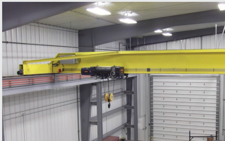
811 Series Compact Conductor Rail on the Cross Bridge
